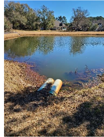
Photo 14 - System Outlet to Pond
